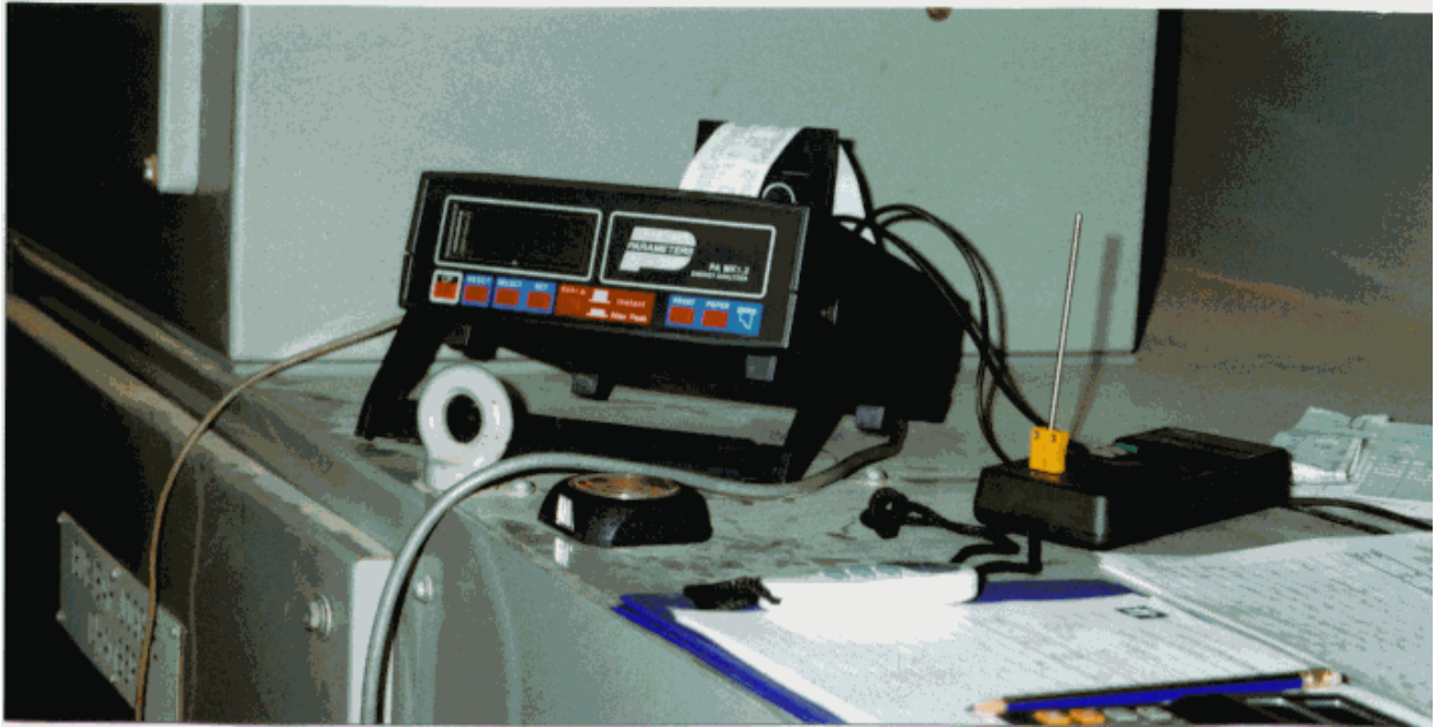
Photograph 1 shows the Microvip connected to the switchboard of a genset during a test.
