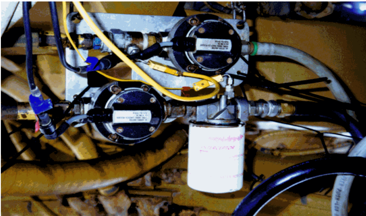
Photograph 3&4 show two flow transducers connected into an engine's fuel lines and the Minitrol Totaliser in operation.
