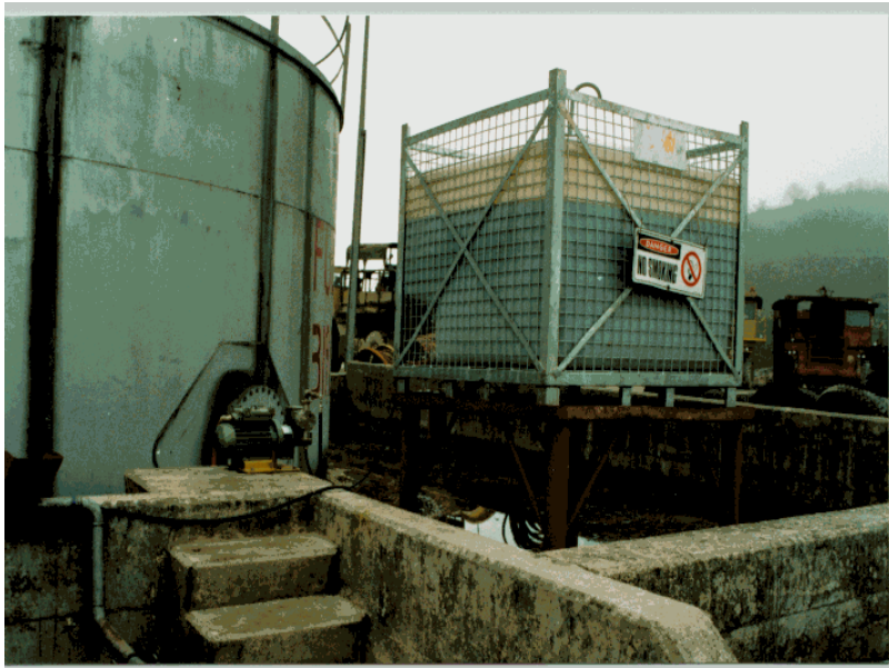
Flow switch activated dosing pump feeding from 1000 litre bulki- box
