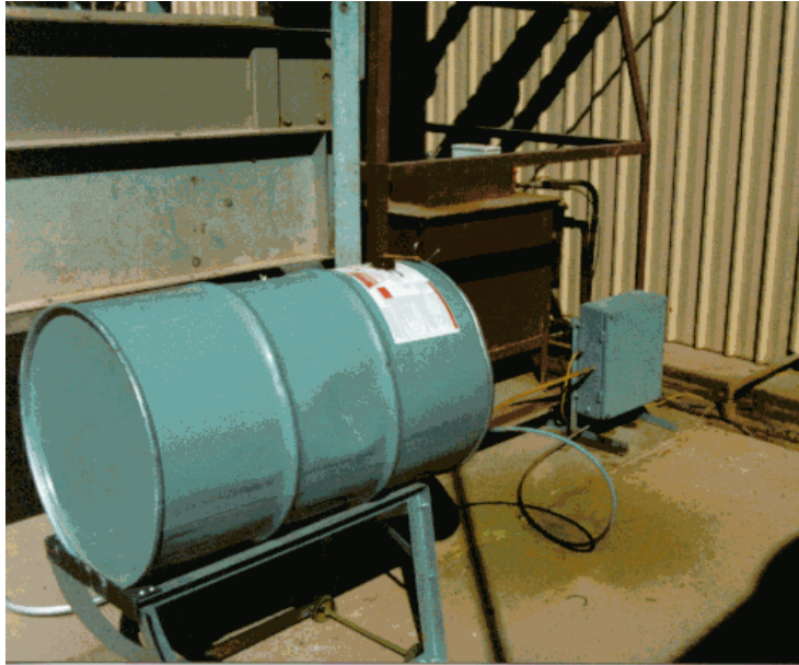
Air operated dosing unit feeding from drum mounted on drum rack
