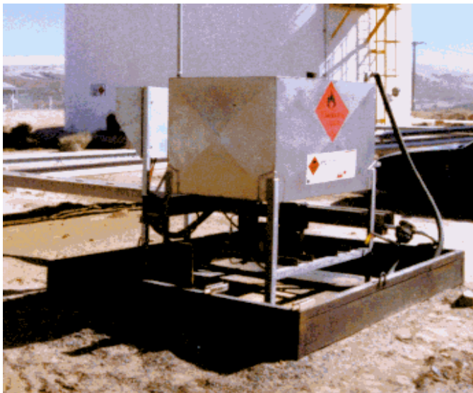
Fully automatic dosing system with 750 liter stainless steel bulk holding tank
